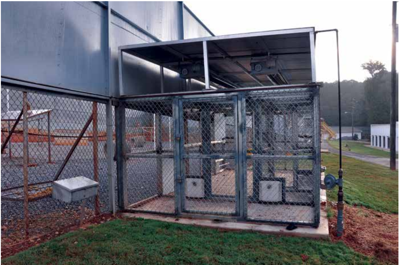
Figure 1. Original introduction enclosure retrofitted with heaters (hanging under the solid roof).
