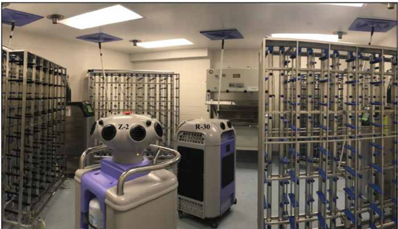
Figure 3. The flex room where assembled IVC racks connected to AHU were VHP exposed in the active–closed setting, with AHU set to the VHP cycle, during months 6 through 12. All equipment required for a scheduled housing room change-out in its entirety was VHP decontaminated the day before by using the Z2 generator and R30 accelerator. Other portable equipment (here, an animal transfer station with its work surface propped open) was VHP decontaminated in the flex room also.
