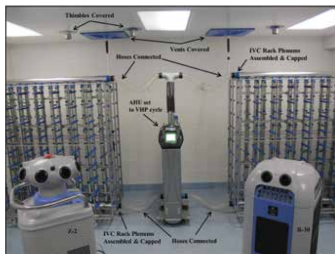
Figure 5. Active-closed VHP exposure, with ceiling thimble connections and HVAC supply and exhaust vents covered, the IVC rack fully assembled, plumens capped, and hoses connecting each IVC rack to an AHU set to the VHP cycle.
