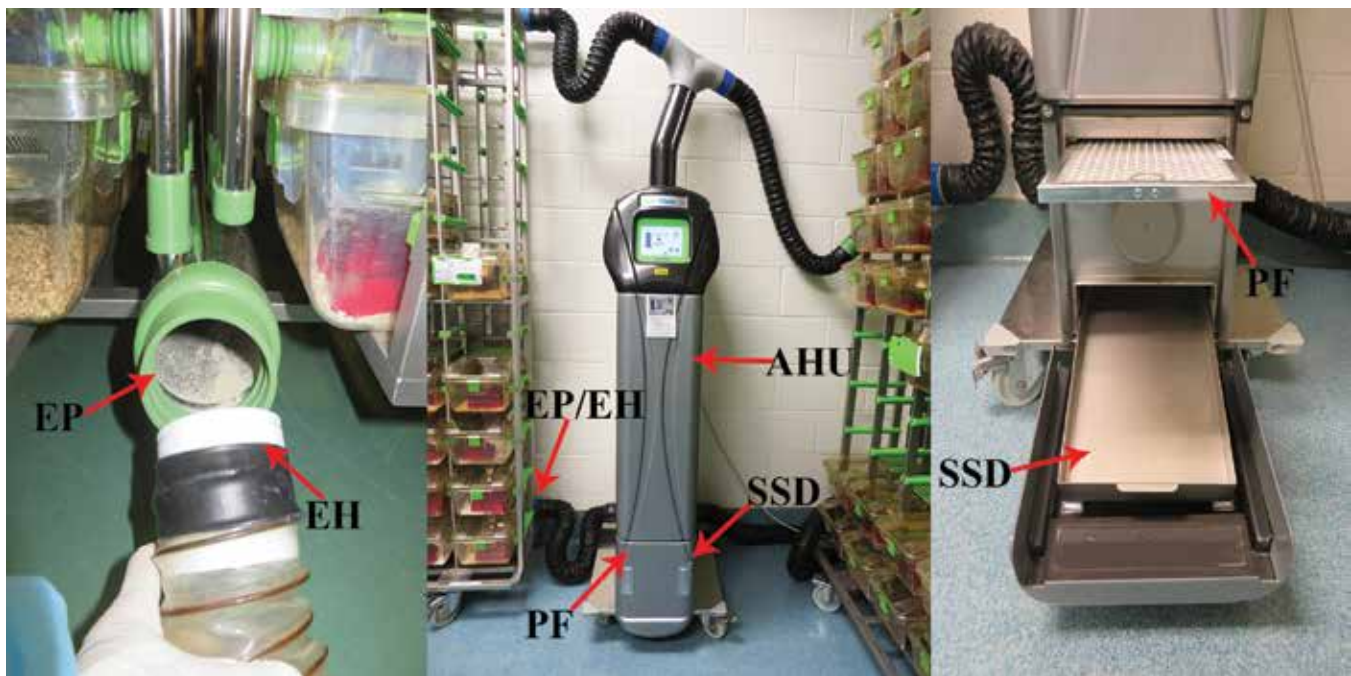
Figure 7. The 4 sites for exhaust air dust (EAD) swabbing on Tecniplast Smartflow air-handling unit (AHU) and Green line IVC rack are shown as: EH, the inside of the exhaust hose connected to the exhaust plenum of the IVC rack leading to AHU; EP, the inside of exhaust plenum at the bottom of the IVC rack; PF, the underside of the exhaust prefilter; and SSD, the stainless steel drawer below the exhaust prefilter.
