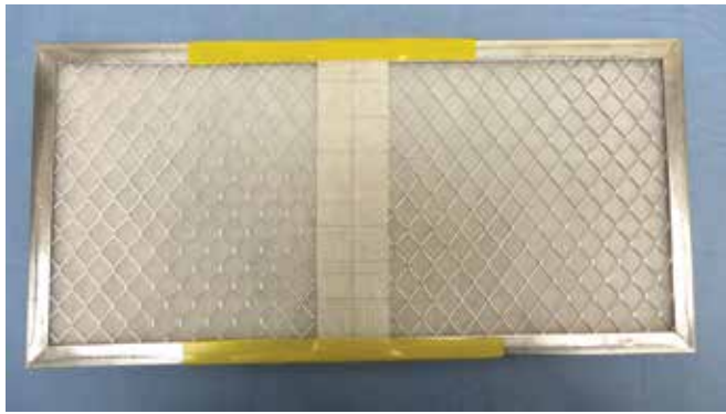
Figure 5. View of the underside of the exhaust prefilter in the air handling unit. A 4 × 18 cm strip of 3M Filtrete 1900 filter paper, with 2 × 2-cm marked squares, was affixed with tape on the underside of the exhaust prefilter.
