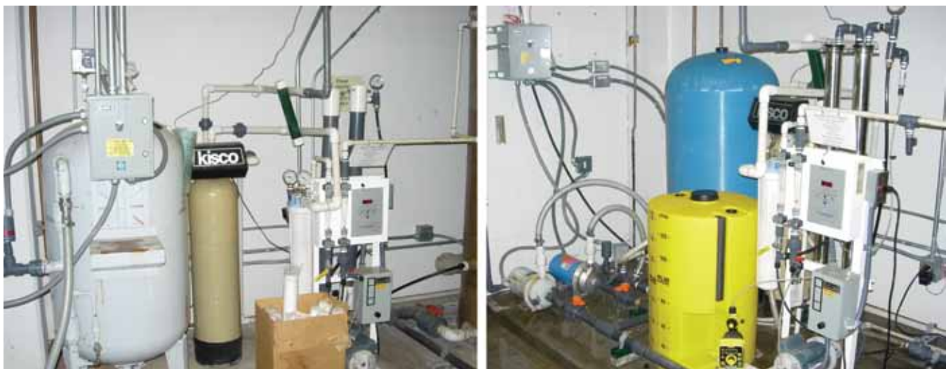
Figure 3. Distribution system before (left) and after (right) modifications. The rubber-lined bladder tank on the old system (gray) was replaced by a fiberglass tank (blue). This modification required moving the nearby electrical box. A chlorine tank (yellow) was added to the remodeled system so that this product could be used as a biocide.
