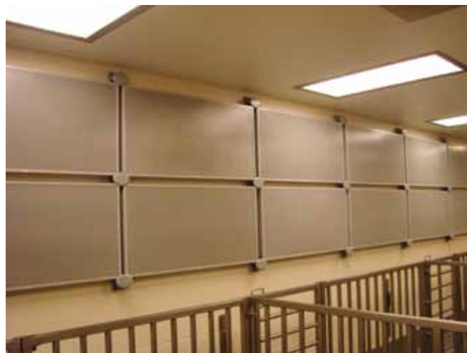
Figure 1. Noise abatement tiles within the hogwash room.
